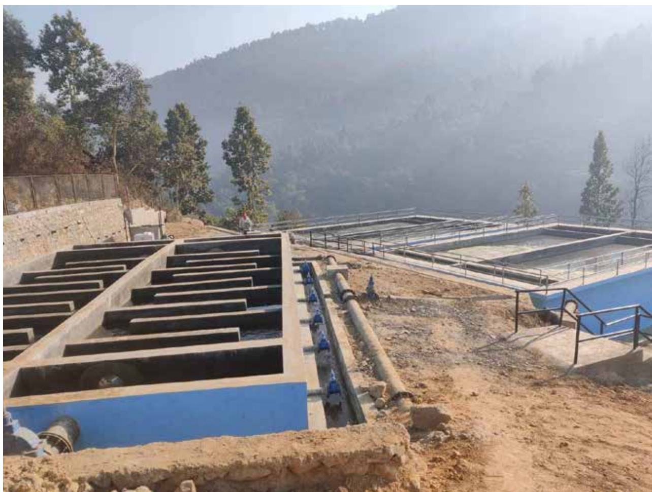
Treatment Plant in an ADB funded water supply project.
